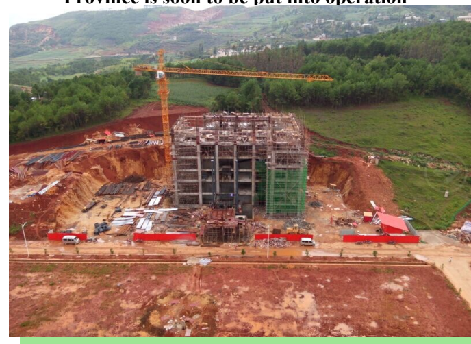
Panorama of the waste incineration project under construction in Baoshan of Yunnan Province
